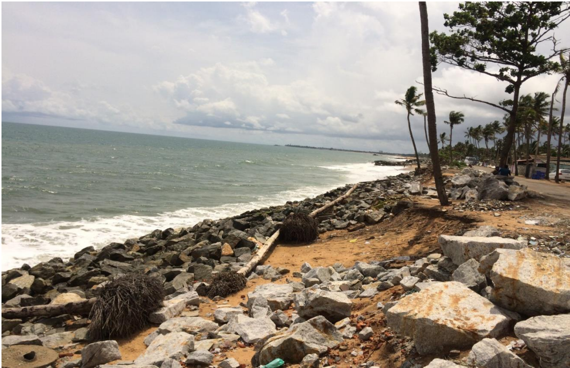
Eroded Coast Eravipuram
