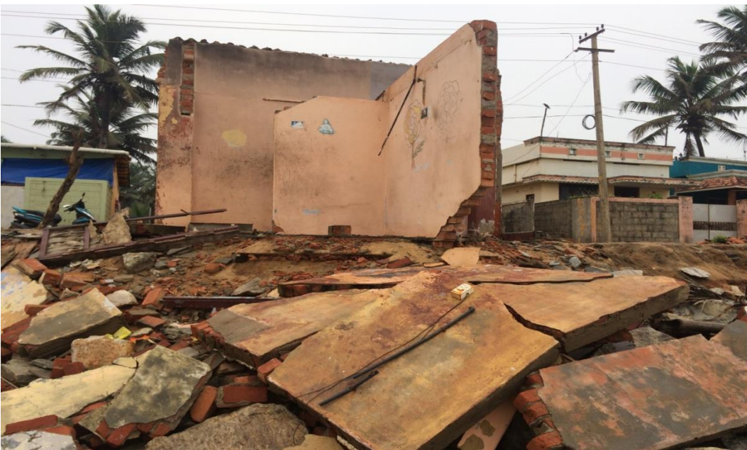
House damaged by Erosion in Eravipuram
